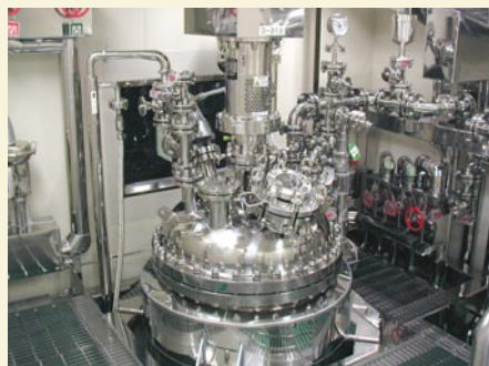
Manufacturing equipment for active pharmaceutical ingredients under clinical trials (class 100,000 clean room)
