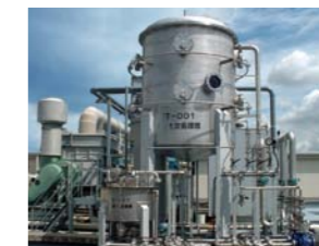
NOx Recovery Equipment
