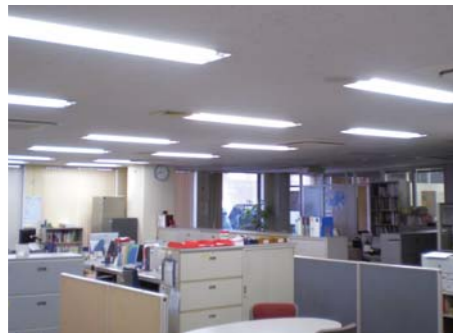
LED lighting has been adopted on a trial basis at a portion of Tokyo headquarters. Data is being collected in order to expand the use of LED lighting.
